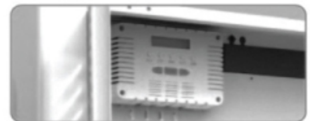
Surge protected power strip and sequenced charge time control. All electrics are UL listed.
